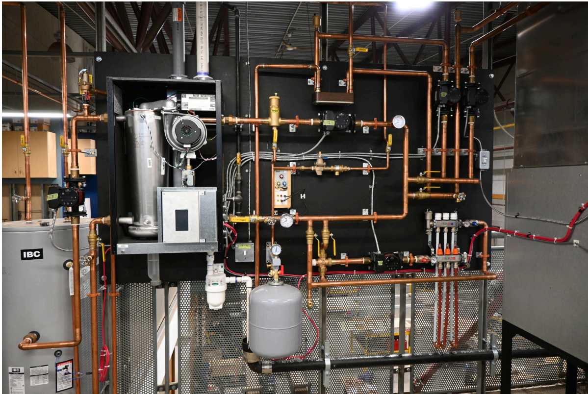
Figure 11 Boiler with piping. (TRU Open Press) CC BY-NC-SA ( https://creativecommons.org/licenses/by-nc-sa/4.0/deed.en )
