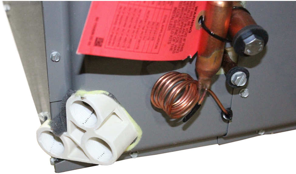
Figure 10 Condensate drain for a cooling fan coil.
