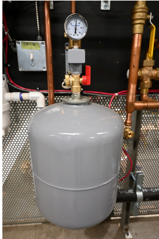
Figure 20 Hydronic expansion tank. (TRU Open Press) CC BY NC SA ( https://creativecommons.org/licenses/by-nc-sa/4.0/deed.en )
