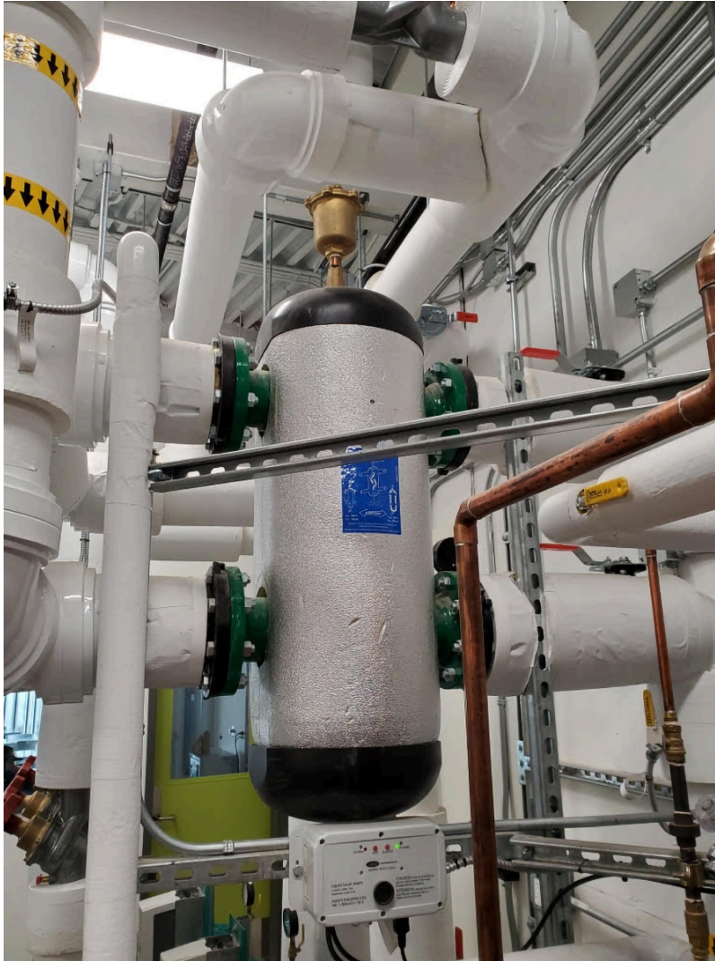
Figure 13 Hydraulic separator. (TRU Open Press) CC BY NC SA ( https://creativecommons.org/licenses/by-nc-sa/4.0/deed.en )
