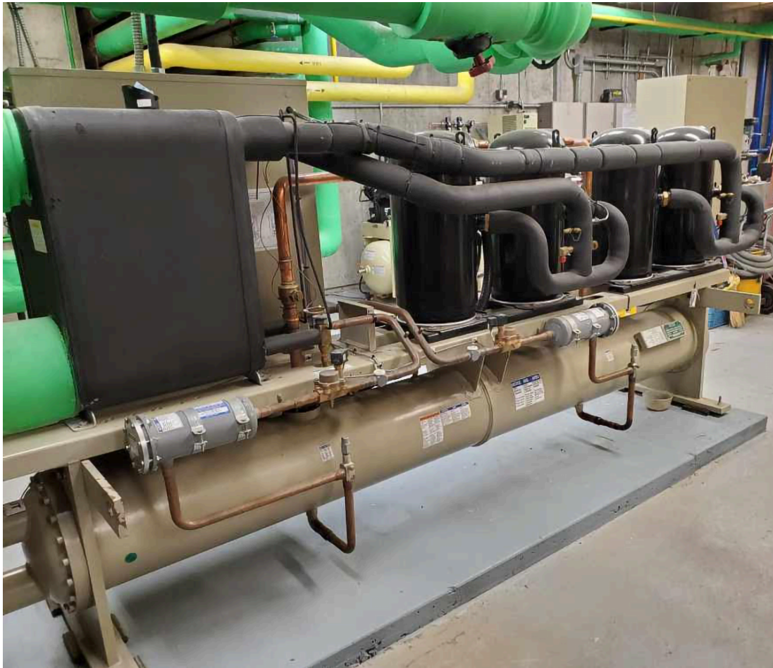
Figure 26 Water-cooled chiller. (Skilled Trades BC, 2021) Used with permission.
