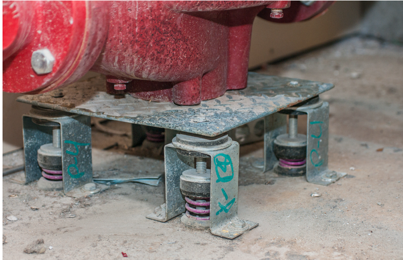
Figure 10 Vibration mounting brackets. (Skilled Trades BC, 2021) Used with permission.
