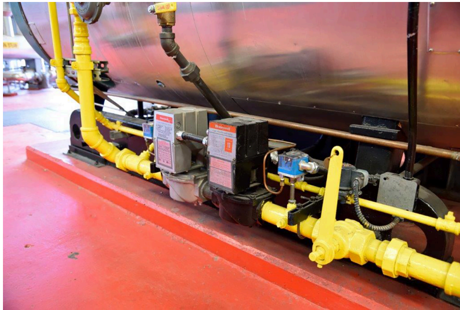
Figure 1 Industrial boiler mounted on housekeeping pad. (Skilled Trades BC, 2021) Used with permission.
