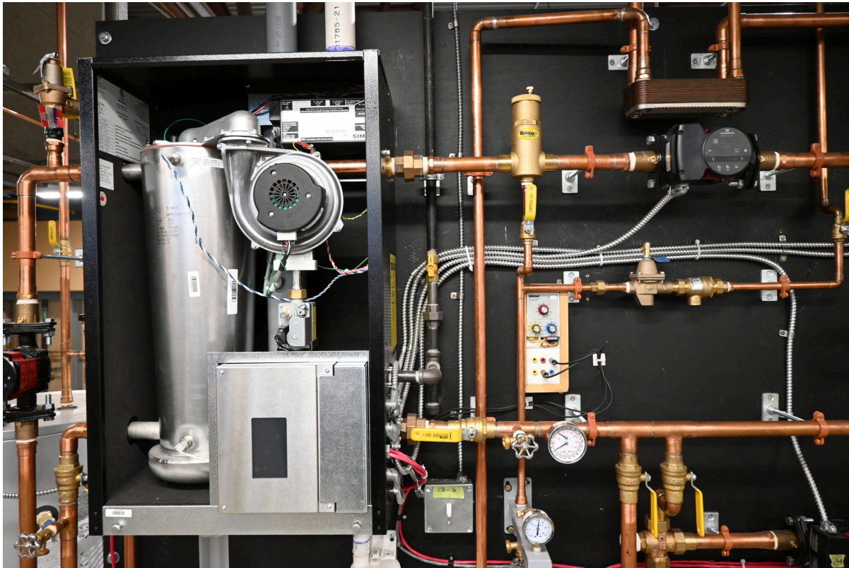
Figure 9 Wall-hung boiler service valves. (TRU Open Press) CC BY NC SA ( https://creativecommons.org/licenses/by-nc-sa/4.0/deed.en )
