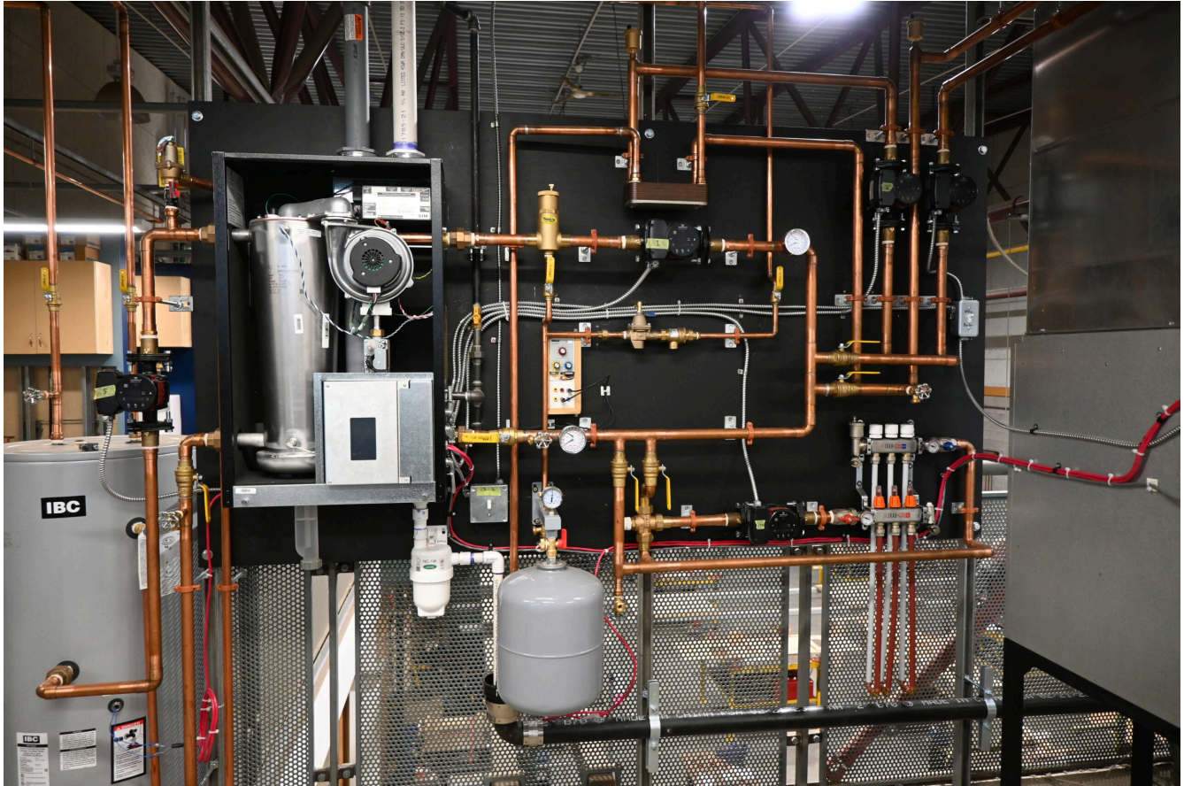
Boiler with piping. (TRU Open Press) CC BY-NC-SA ( https://creativecommons.org/licenses/by-nc-sa/4.0/deed.en )
